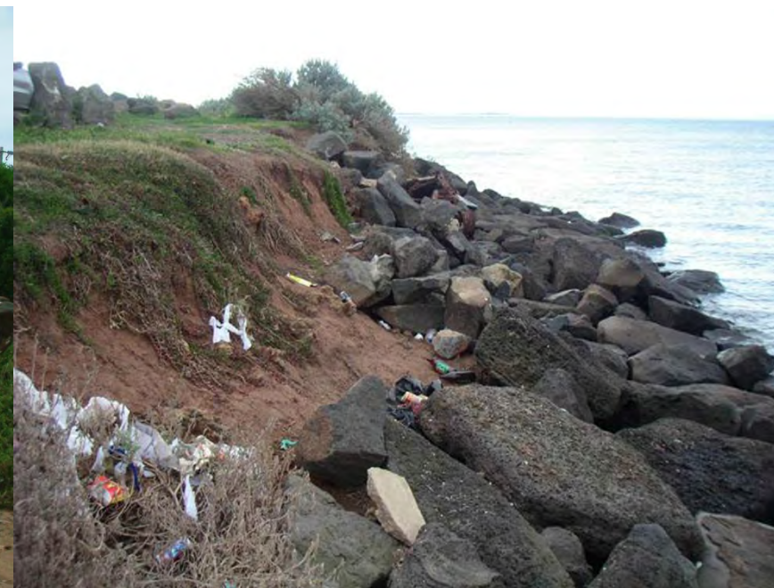
Erosion behind the rock armour along the coastal bluff
